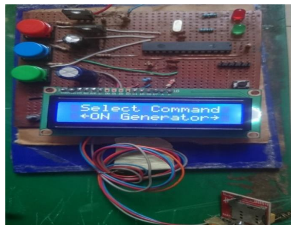
Figure 9: Menu to Switch ON the Generator
