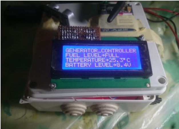
Figure 15: Status of Generator of When Temperature above Rated Maximum Value and Fuel Level is Full
