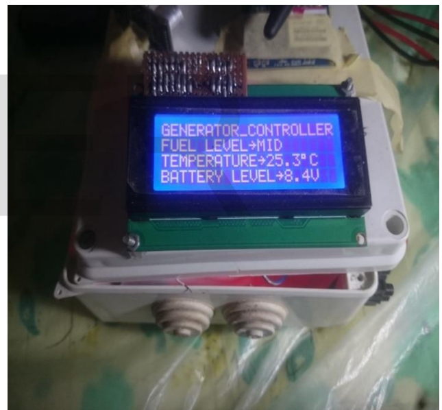
Figure 14: Status of Generator of When Temperature below Rated Maximum Value and Fuel Level is Middle
